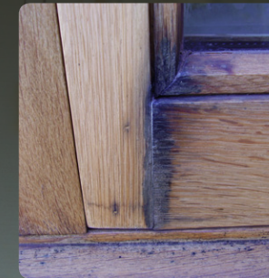
Example of tannin staining on an oak window
